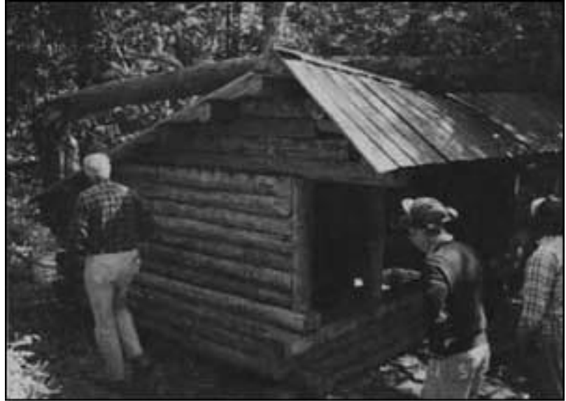
Members of the Connecticut Chapter of the Appalachian Mountain Club inspect the damage to the Limestone Springs Shelter.
