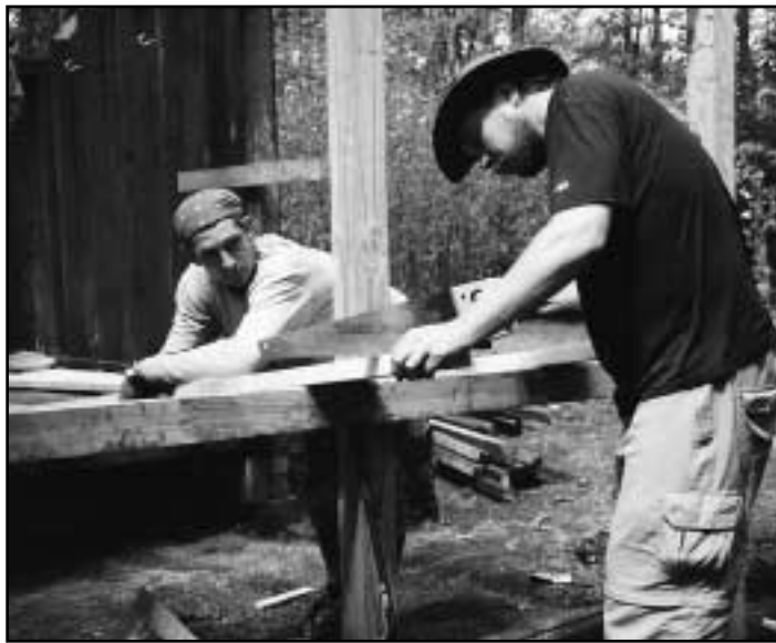
Damascus Hard-Core crew reroofs the Clyde Smith Shelter and constructs a cooking-pavilion extension. (ATC photo by Laurie Potteiger)
