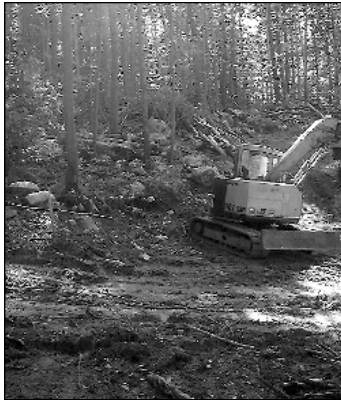
Construction encroaching on A.T. lands near Great Barrington, Massachusetts. (Photo: Cosmo Catalano)
