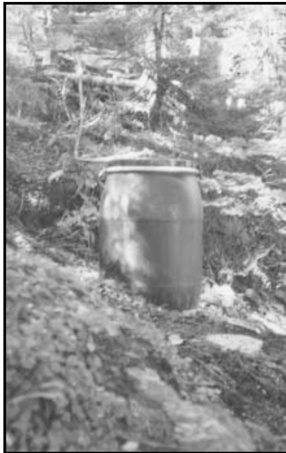
Figure O.2—The beyond-the-bin liquid filter barrel at Taft Lodge. The barrel contains anthracite coal and washed septic stone and drains out from the bottom into the soil, once filtered. (Photo by Pete Ketcham)
